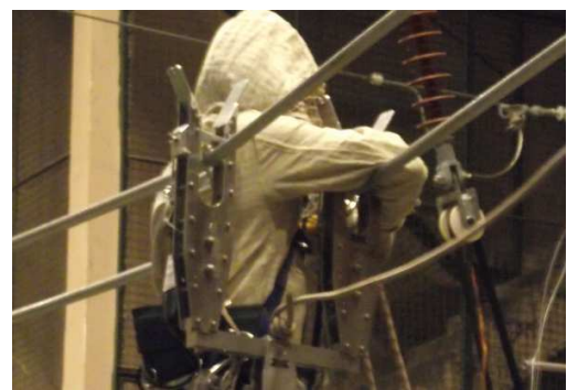
Figure 7: live-line maintenance with conductors close to the worker's head
